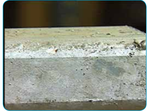
Dross Inclusions (acceptable unless large and if removed, a bare spot is exposed)
